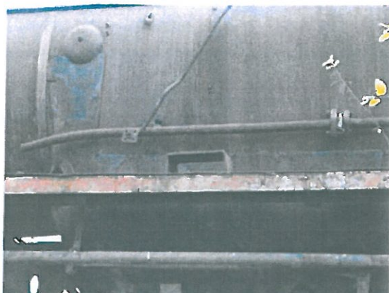
Ty2-1226 Fundament turbogeneratora
